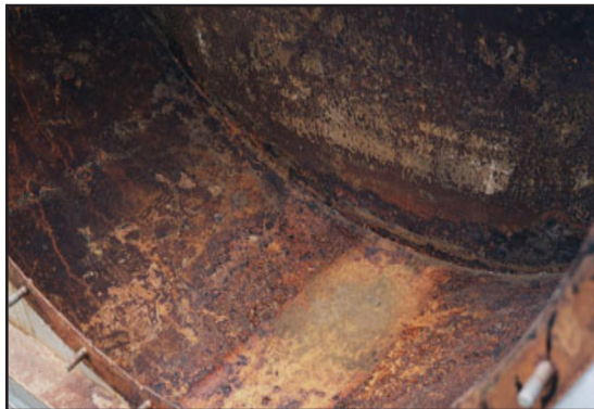
Inside the housing after FRP removal
